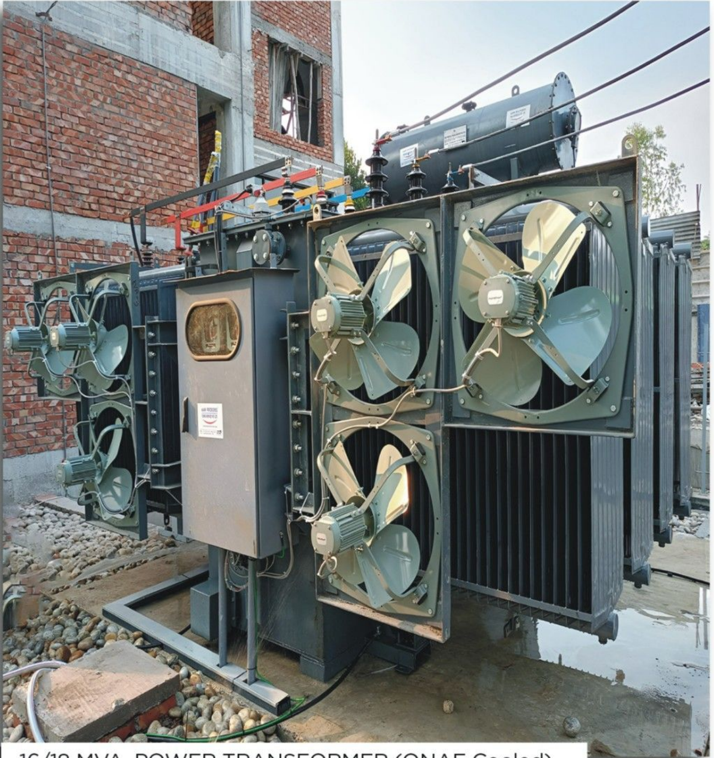
16/18 MVA, POWER TRANSFORMER (ONAF Cooled)
